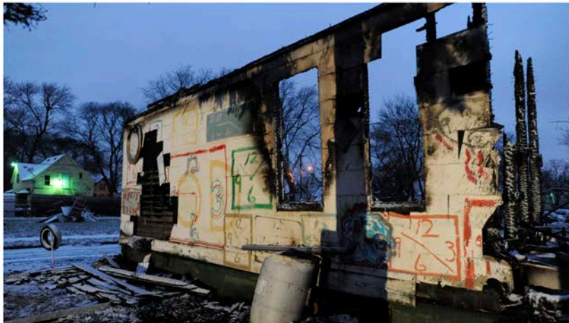
A partial wall is all that remains of the Clock House on Dec. 9, 2013. The roof collapsed, leaving only charred timbers from the foundation.
