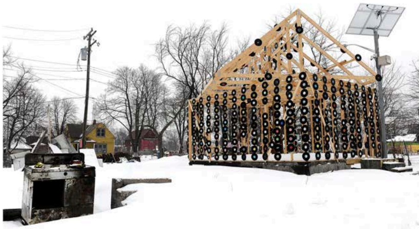
A stove that was inside the Heidelberg House of Soul sits outside the framework for a new house being built in the same location. The original House of Soul was torched in November 2013.
