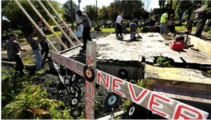
UAW Local 412 volunteers raise the first wall of the House of Soul on Sept. 27, 2014. The volunteers helped rebuild the house that was destroyed by arson in 2013.
