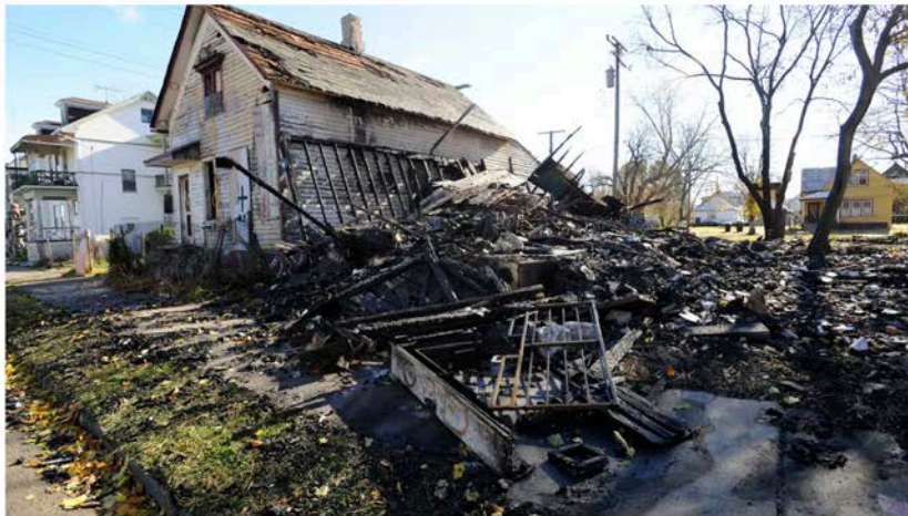
The aftermath of the fire at the House of Soul leaves a charred mess at the Heidelberg Project on Nov. 12, 2013.
